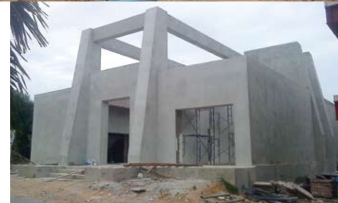
Above: The Japanese House is nearing completion. Top: Progress at Suan Suwarn 1. Facing page (top): The I-boutique condominium. Far left: Latest picture of Park Royal.
